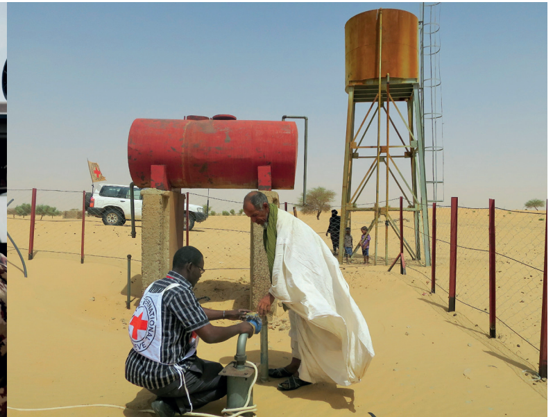
The Village Chief of Likraker in the Tumbuctu Region of Mali inspecting the reconstructed drinking-water plant. The rehabilitation work benefits 1,200 inhabitants and their livestock herds.
